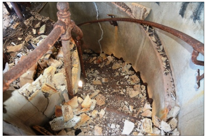
Deteriorating condition of lighthouse staircase. The bottom of the lighthouse was worse, with several inches of debris, plus trash left behind over the years.
